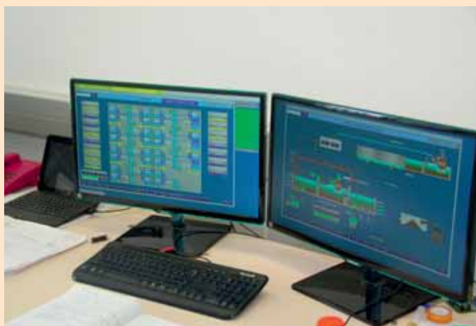
While many of the processes in the hatchery are automated, human monitoring plays a critical role in keeping mortality rates manageable.
